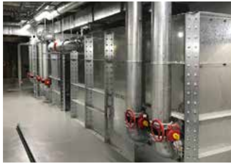
Waratah Place rectangular tanks
