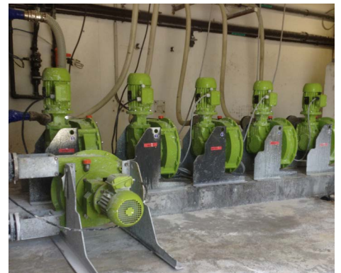
ALHX40 for lime slurry in wastewater treatment
