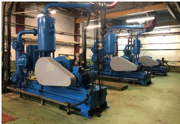
ABEL HM pump at a wastewater treatment plant
