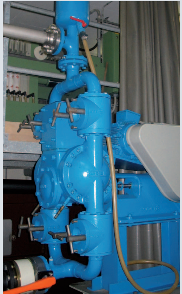
Ball valves with inspection opening and membrane leakage detection device
