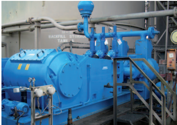
ABEL HMT for transfer of concentrated copper tailings
