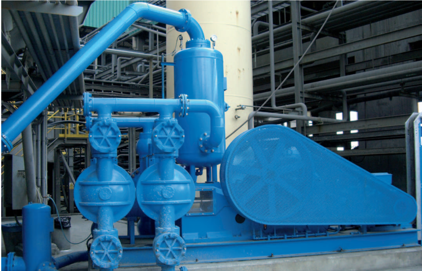
ABEL HMQ for tailings transfer in a copper/nickel mine
