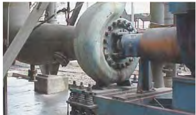
Model 3180XL on difficult high temperature service. Spring-mounted baseplate provided to compensate for thermal expansion.
