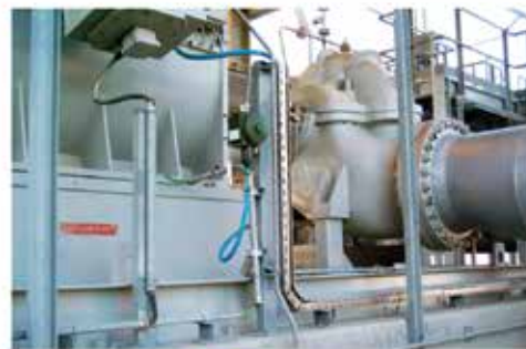
Refinery Crude Oil Service (Middle East)
