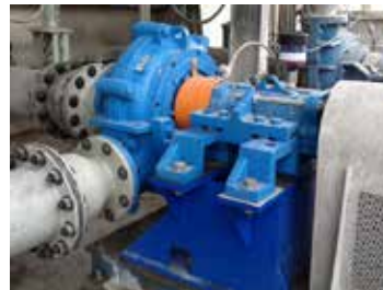
Ball mill discharge in Phosphate plant
