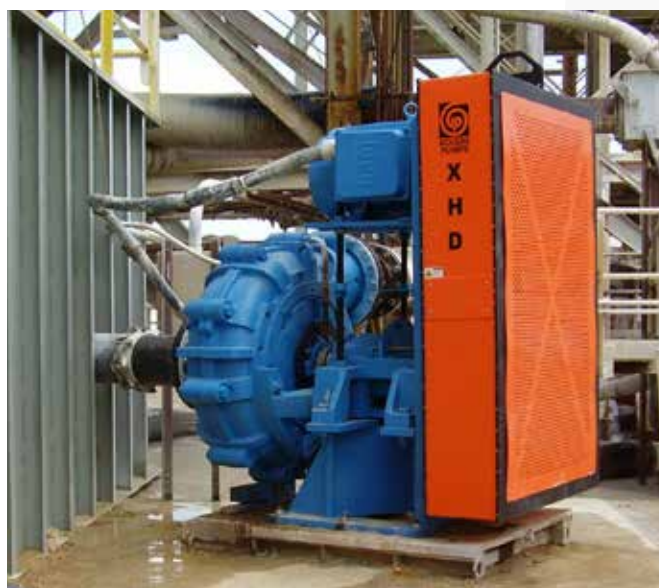
Primary Sand Slurry Pump in an Aggregate Plant
